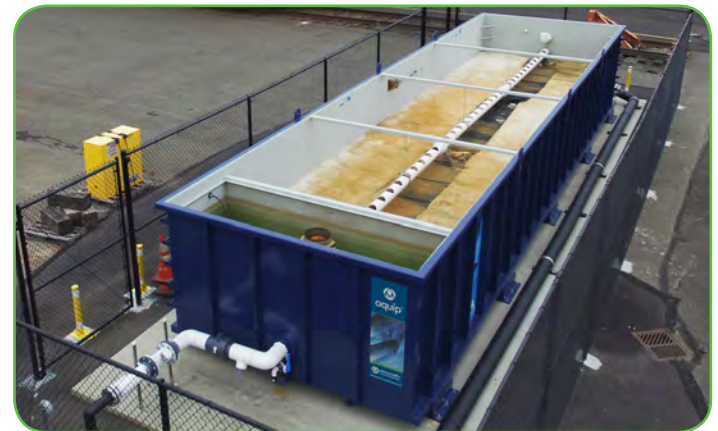
Aerial view of an AquiP 400 system
