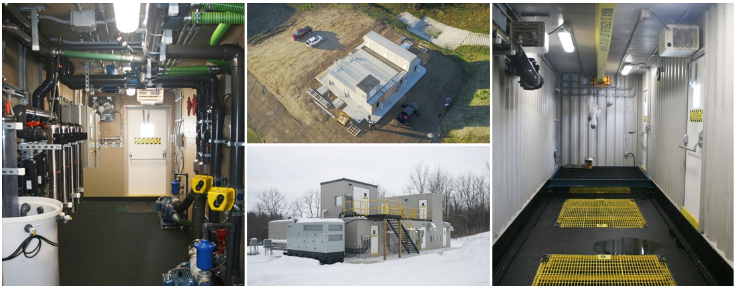
The Newterra fully-clad system in the small Township of Southwold, came complete with odor & noise attenuation, due to its proximity to the development and surrounding green space. The first system was designed with a capacity of 500 m 3 /day (132, 000 GPD), with the option of being expandable to 317, 000 GPD (1,200 m 3 /day).
